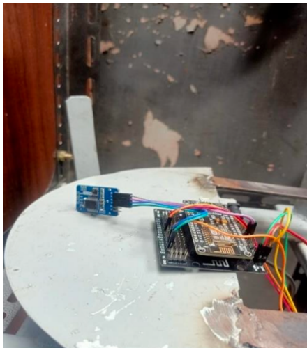
Fig 3. Sensor and ESP8266 installation
